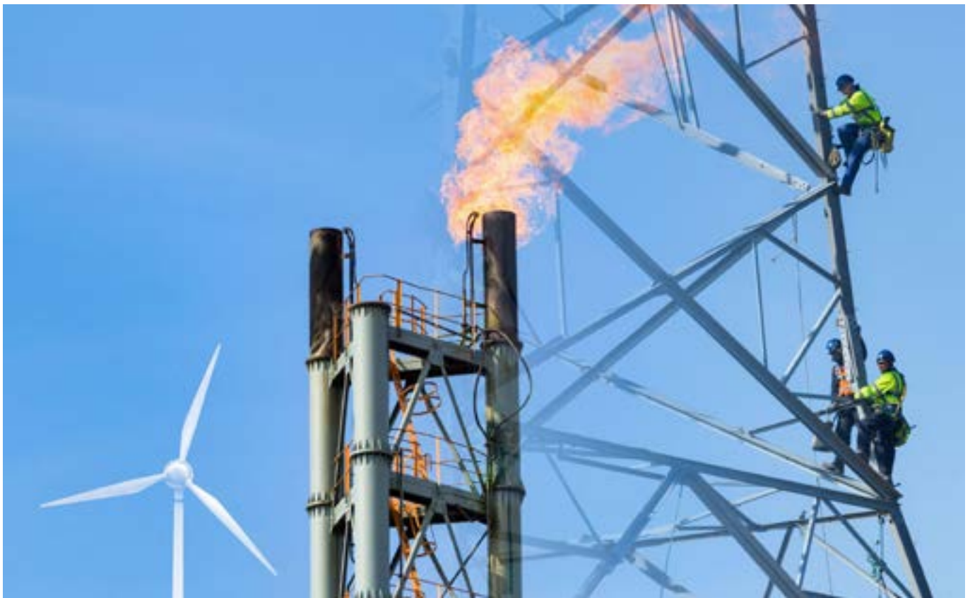
National Grid gas distribution operations
